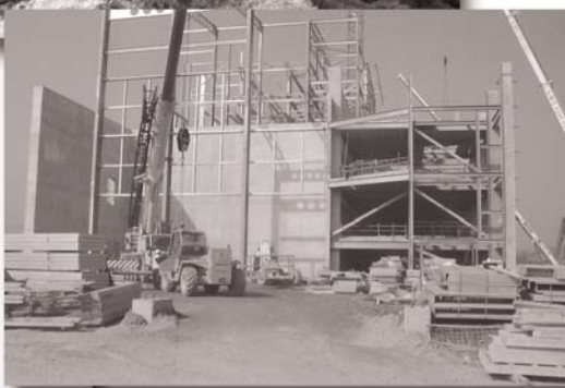
The new incinerator
